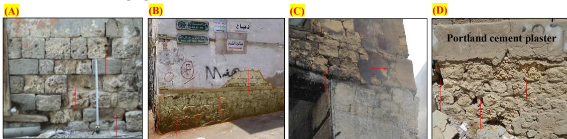
Figure. 14: Photos illustrate the weakness and deterioration of the external leaves constituent materials.
