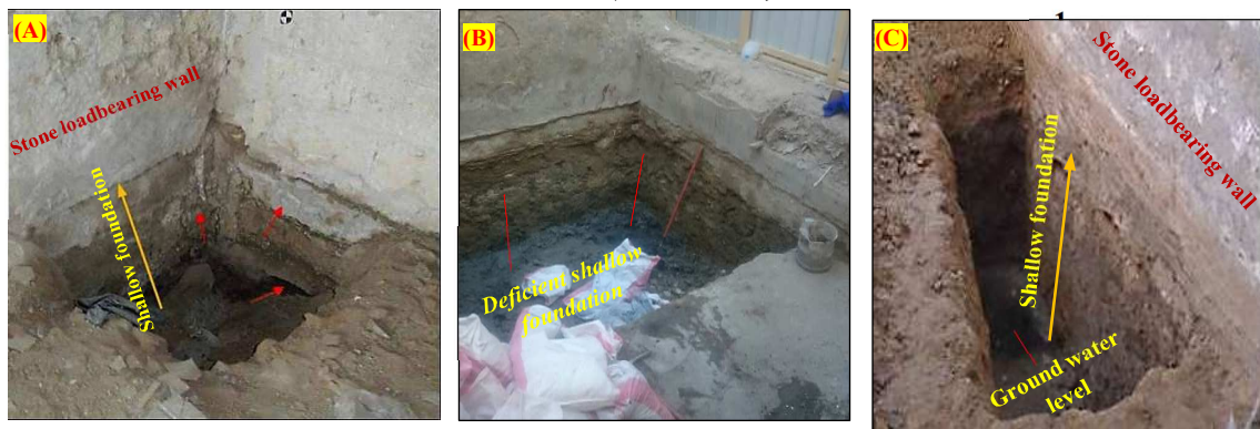
Figure 6: (A, B) Illustrate the vulnerability of the structural state of the shallow foundations of heritage buildings in historic Jeddah; (C) shows the ground water rise and its leakage to the foundation.
