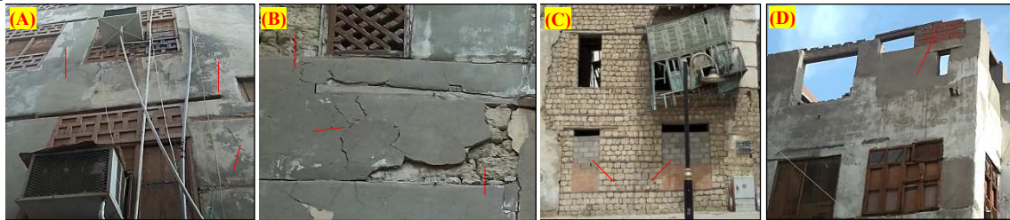
Figure. 16: Shows the effects of the use of incompatible building materials; (A, B) black cement plaster (Portland cement); (C, D) red bricks and sand crete blocks.
