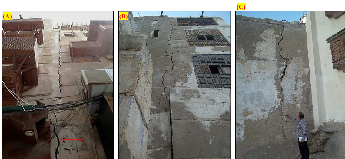
Figure. 7: Large vertical structural cracks run through the entire height of the masonry walls of some heritage buildings at historic Jeddah.
